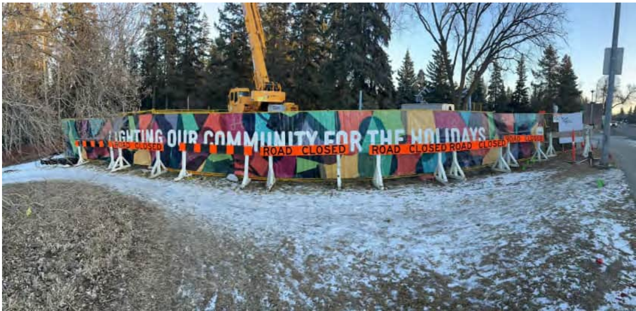
Decorative Art Hoarding installed at 142 Street and Summit Drive as part of the 99 Avenue Trunk Rehabilitation Project
