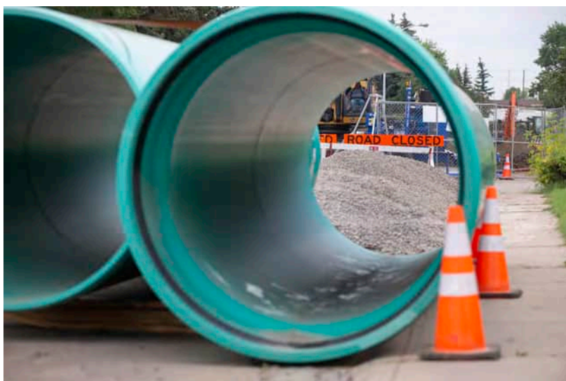
PVC Sewer Pipes
