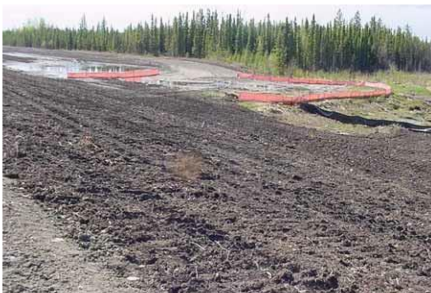
23. Good layout of silt fences in “smiles,” however it appears that seepage has gone around the end of the upper silt fence
