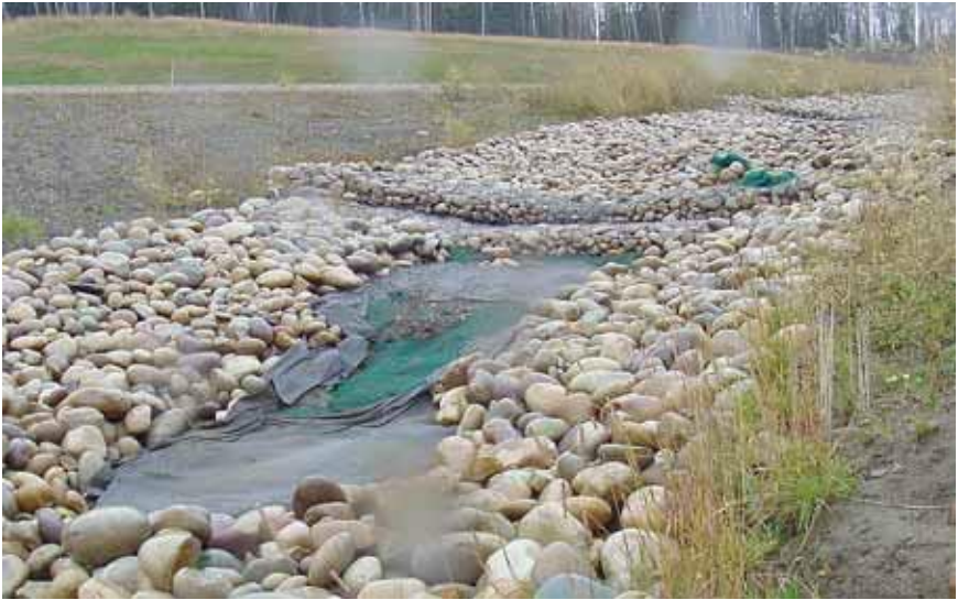
3. Failure of riprap protection. Even riprap requires maintenance. Water washed rocks away and exposed geotextile.
