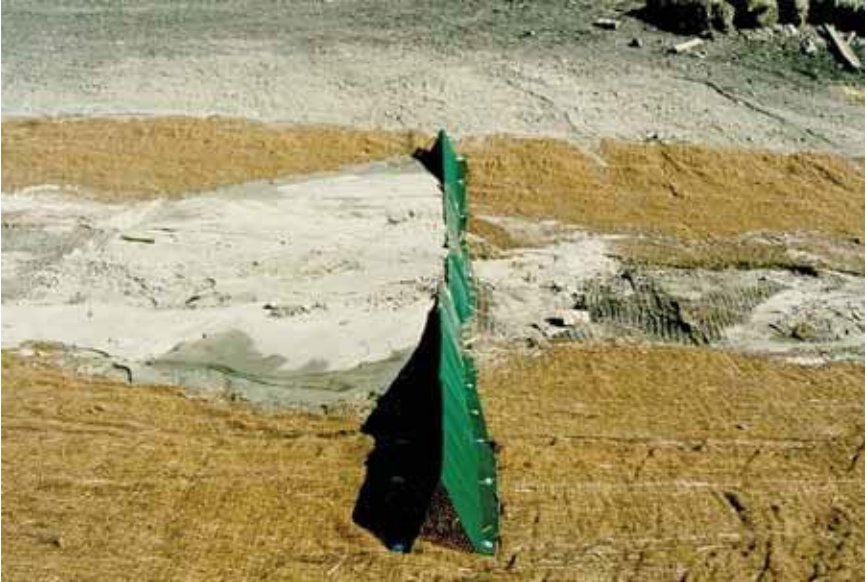
35. Synthetic energy dissipater working well but needs maintenance to remove sediment
