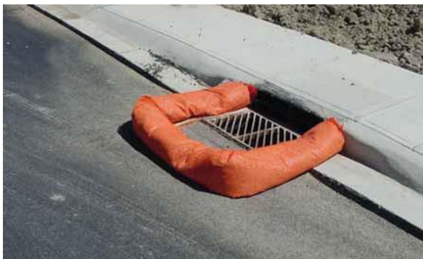
41. Some protection of Inlet, but It needs protection along top of curb
