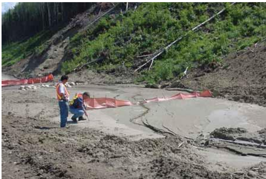
22. Silt fence overloaded to failure
