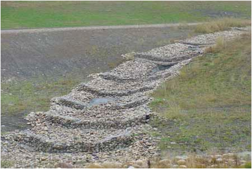
29. Rock check dam. Failure due to scour under geotextile. Water velocities may have exceeded the design velocities.
