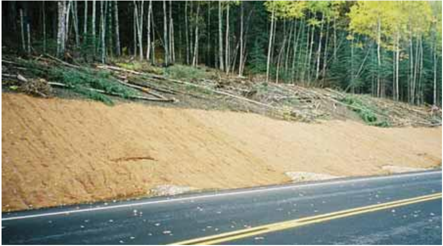
16. Rock ditch checks, erosion control blanket on lower slope and use of cut material to protect slopes on upper slope
