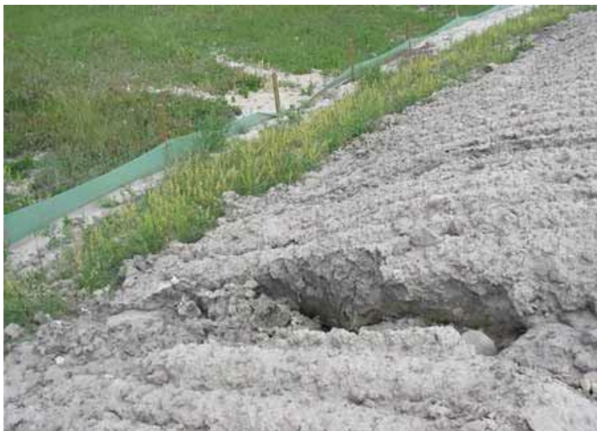
12. Furrowed in the wrong direction. Furrows should be perpendicular to slope
