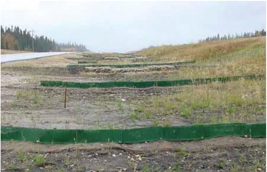
30. Synthetic and rock check dams. Failed due to poor anchors causing flow under synthetic check dam.
