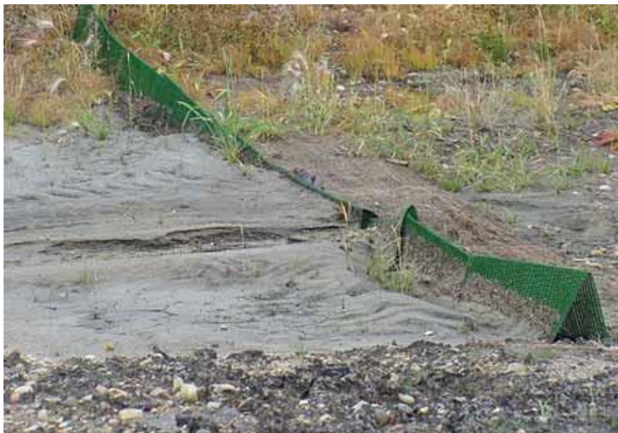
28. Synthetic check dam. Failure due to overtopping and sediment buildup. Check dam separated when flow overtopped structure.
