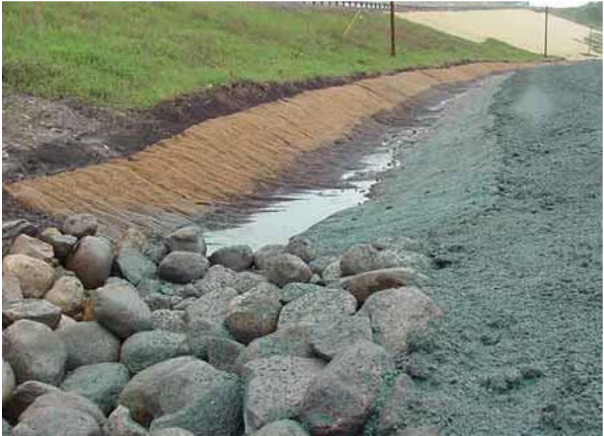
19. Erosion control blanket on top of slope, erosion control mat in channel and riprap for energy dissipation
