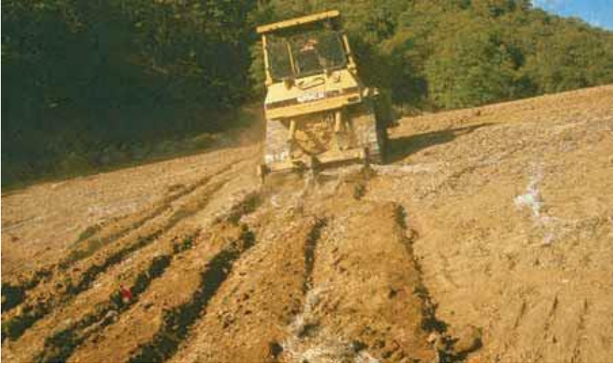
10. Cross furrowing on slope. Watch for low spots where water will collect
