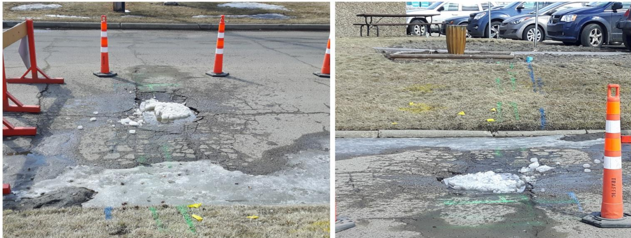
Figure 3.0-1 Active Subsidence around a Failed MH
